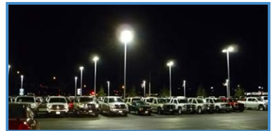
Waconia Dodge installed 32 pole lights and seven wall packs to the exterior of the building.
